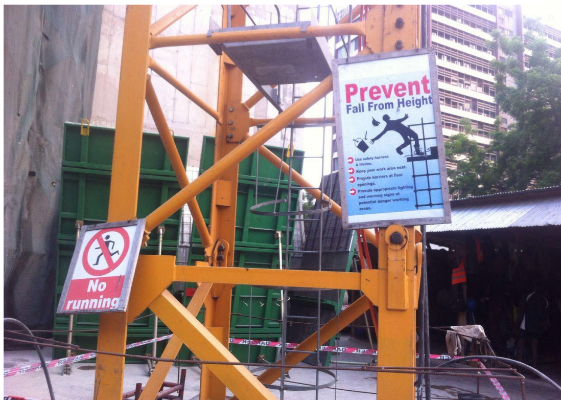
Figure 22: Signages posted on a crane stand to restrain workers from running on site and how to prevent falling from heights.
