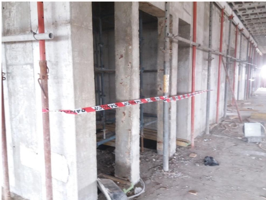
Figure 16: Caution and warning tape wrapped around a floor hole to warn workers of the possible danger.
